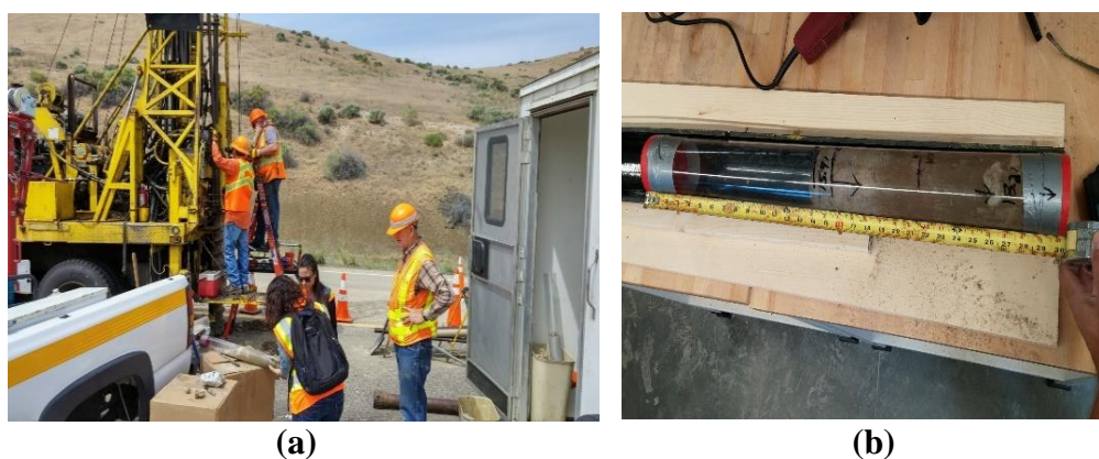
Figure 3.6 Drilling and Sample Collections: (a) Full view of Drilling Operation (b) Plastic Tube Sampler with Soil Sample Inside (Sample Collected in May 2015; Courtesy-ITD)
