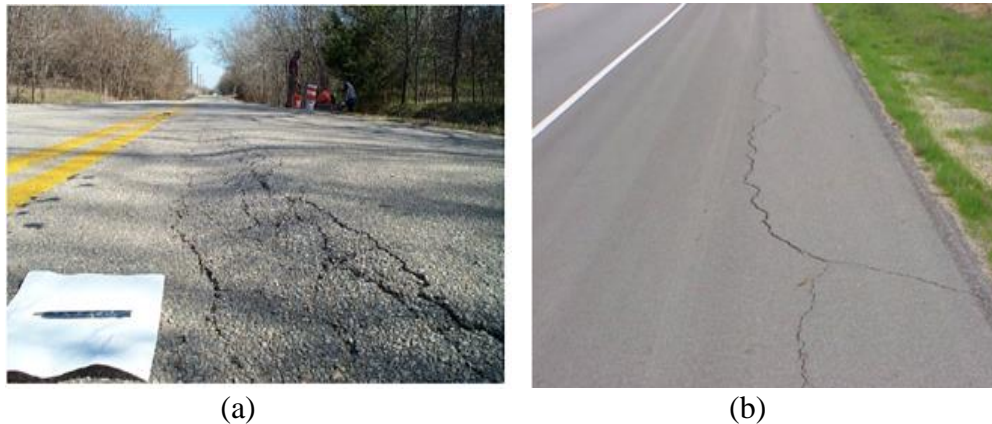
Figure 1.1 Photographs Showing Damage to Pavement Systems due to Volume Change in Underlying Expansive Soil Deposits (Manosuthikij, 2008)
